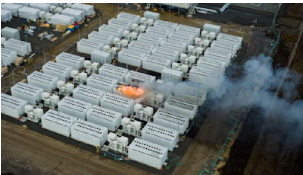
Thermal Runaway – Victoria Big Battery project, Australia
